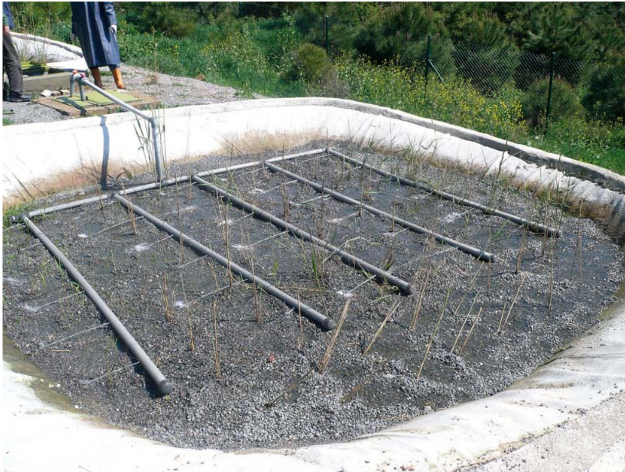
◀ Figure 7: TECHNICAL AND DEMONSTRATION CENTERS HAVE BEEN ESTABLISHED IN FOUR DIFFERENT MEDITERRANEAN COUNTRIES: EGYPT, MOROCCO, TUNISIA AND TURKEY
