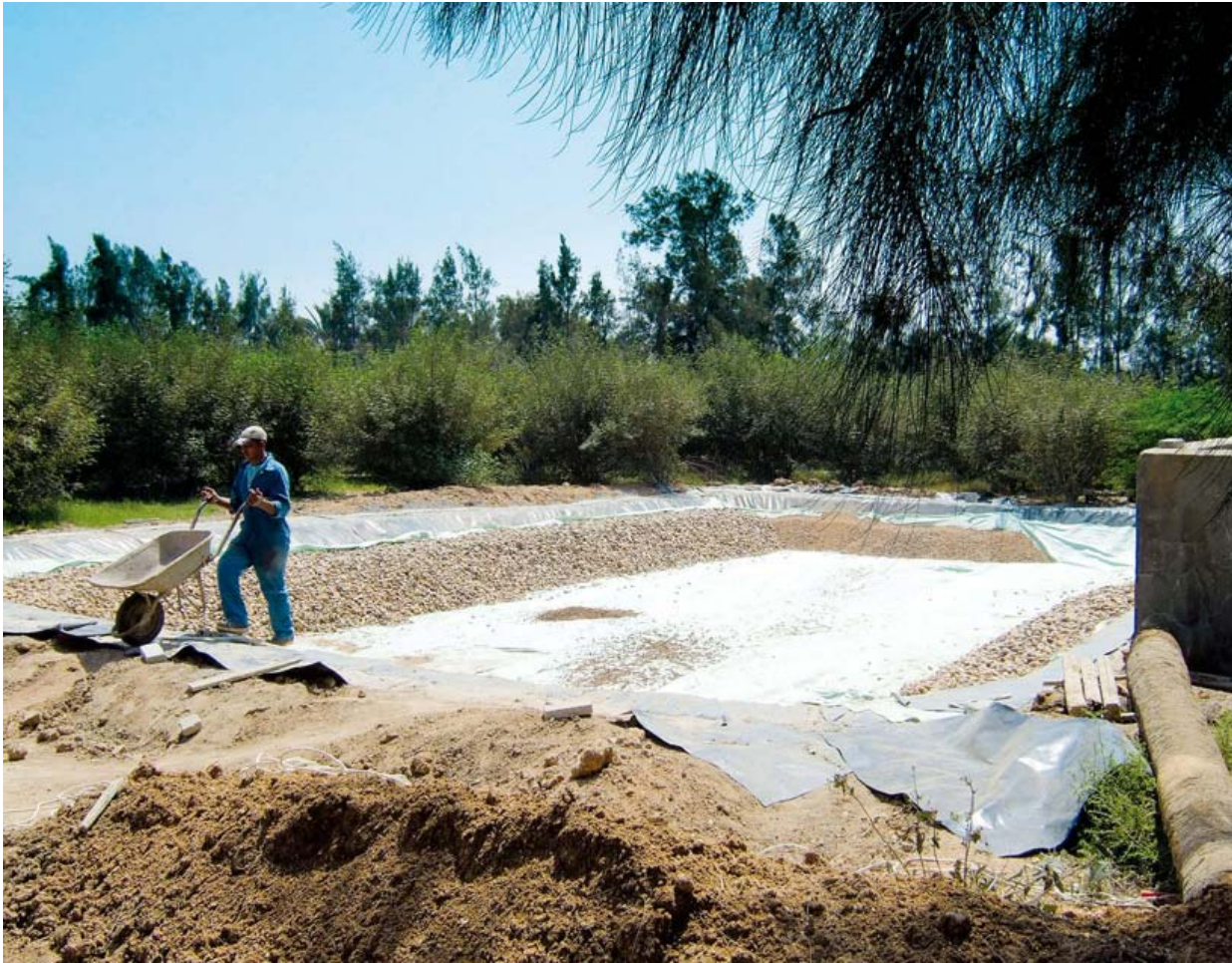
◀ Figure 3: CONSTRUCTED WETLAND FOR PRODUCTION OF IRRIGATION WATER ET SEKEM, EGYPT
