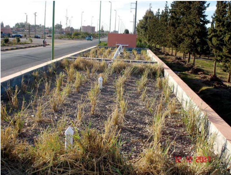
▲ Figure 2: GROWN-UP GREYWATER TREATMENT PLANT FOR THE HAMMAM IN EL ATTAOUÏA
