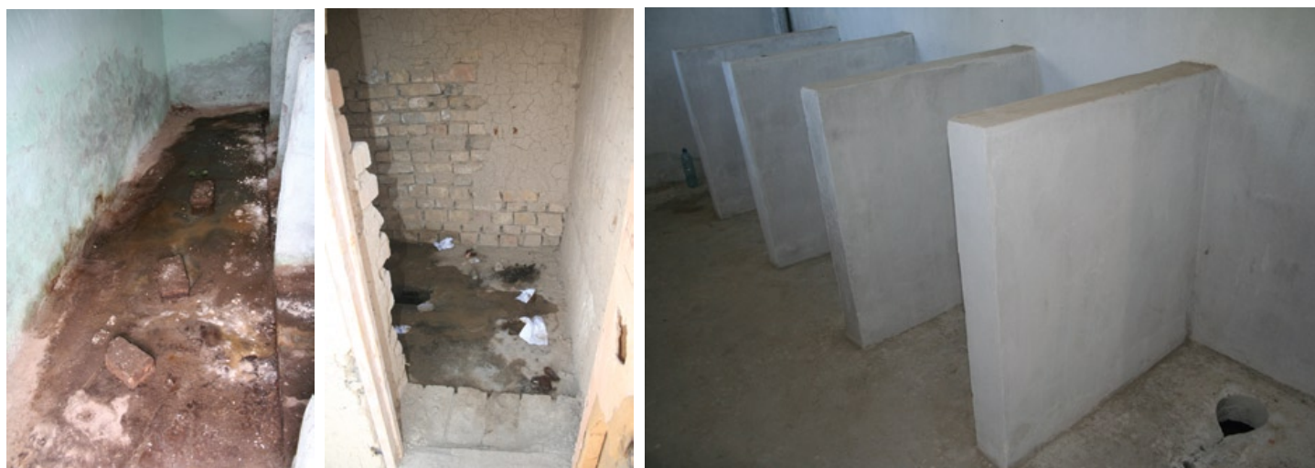
FIGURE 2.3 School latrines, Osh Province, Kyrgyzstan
