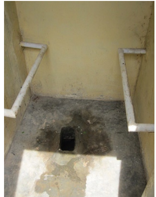
FIGURE 6.6 Disability-friendly latrine in rural Uganda
