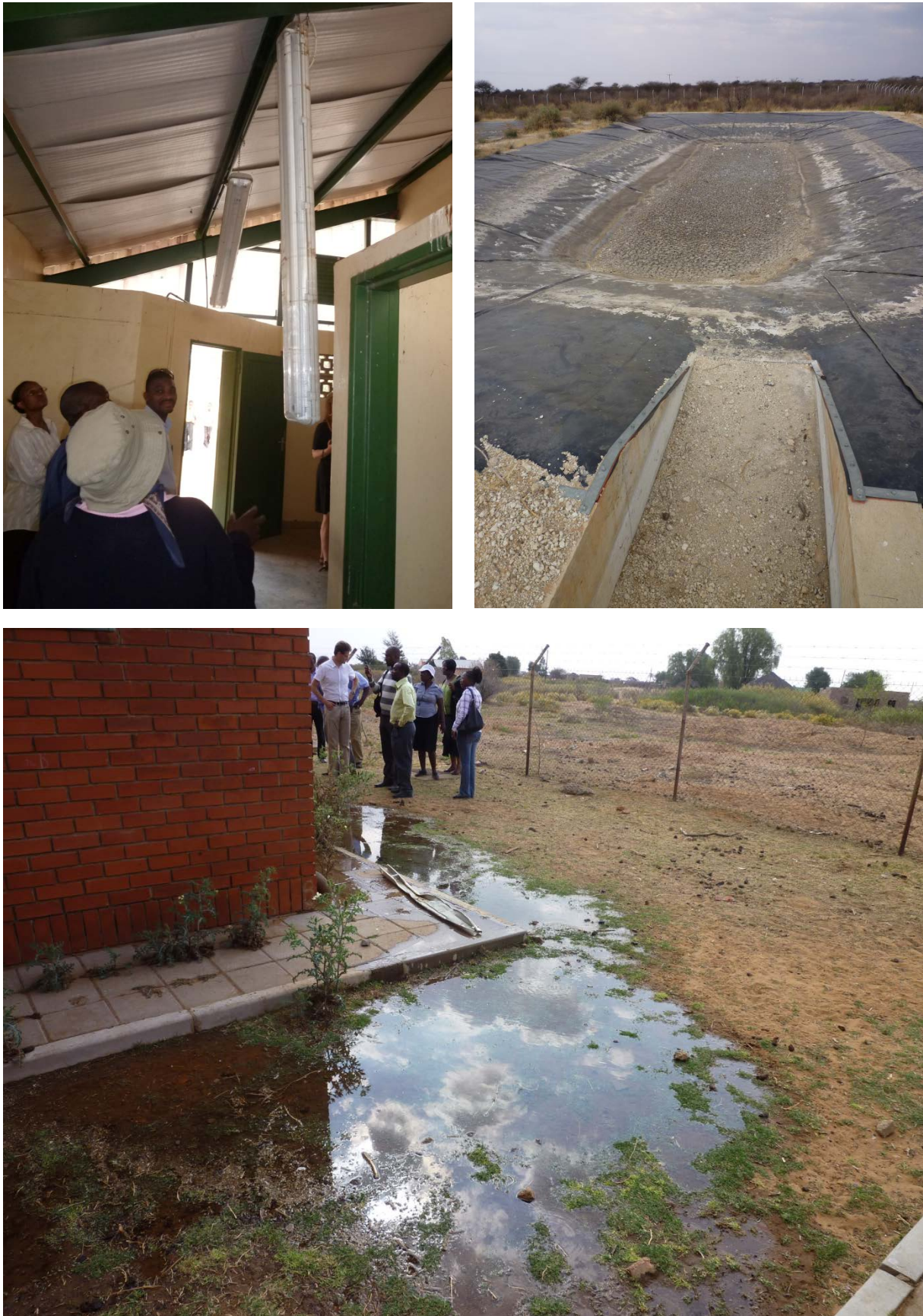
Figure 6. Maintenance problems at institutional facilities encountered during community walk. Top left: vandalized lamps at Letlhakeng Primary School. Top right: empty sewage ponds at Mphuthe JSS. Bottom: leakage caused formation of a large pool of water outside the toilet block.
