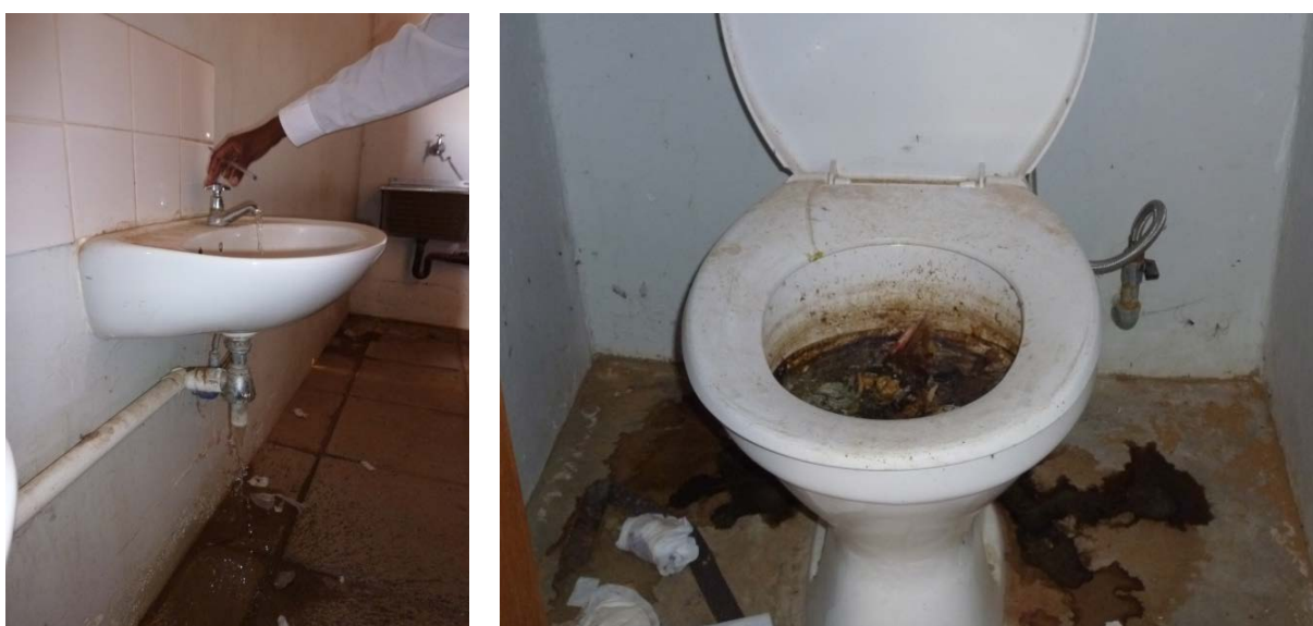
Figure 9. Maintenance issues in Mphuthe JSS toilets: water running from sinks straight onto the ground (left); clogged toilet (right).
