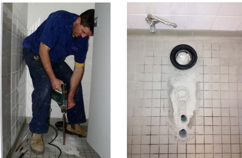
Figure 11 (a) Our plumber drilling the hole for the urine pipe in the 200 mm-thick concrete floor and (b) Holes drilled in the floor for the urine outlets of the Wostman and Dubbletten UDTs
