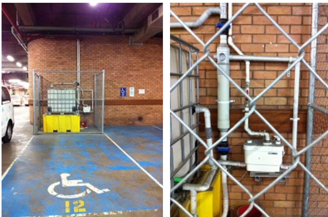
Figure 15: (a) The installed tank (b) The Saniflow pump and urine sampling unit
