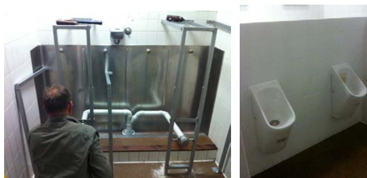
Figure 14: (a) The plumber installing metal framing to the existing slab urinal to retrofit the waterless urinals (b) The retrofitted waterless urinals.
