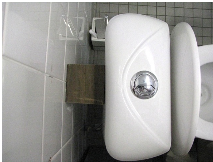
Figure 50: The back of the UDT stands closer to the wastewater outlet than a standard Australian toilet. A image shows the wooden block that was placed in the gap to give stability that the wall would normally have provided to the UDT's cistern.
