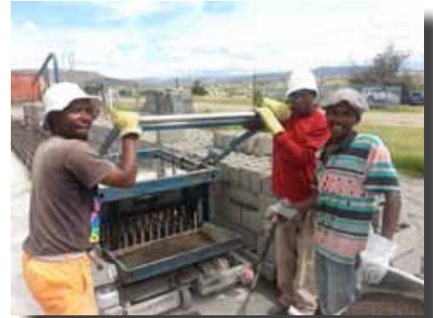
Figure 9: At the Maggie Resha Zone Site a mobile block machine is used, casting blocks four at a time on a large flat slab
