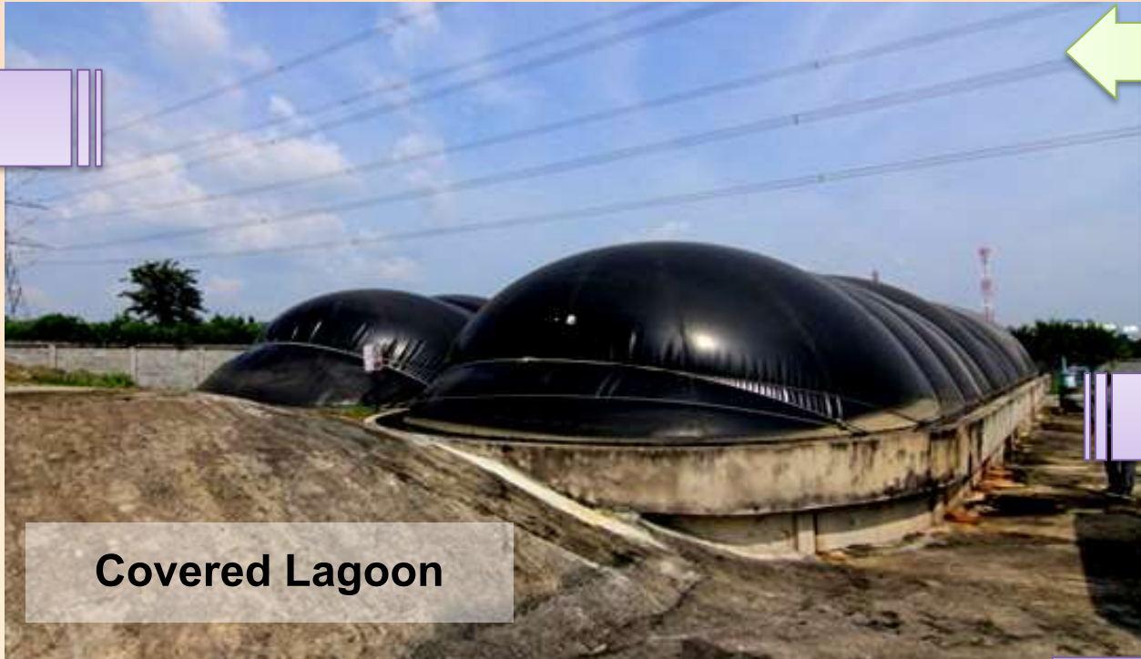
Electricity Generator from Biogas
