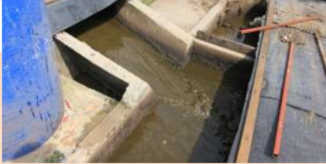
FS flow through screening
