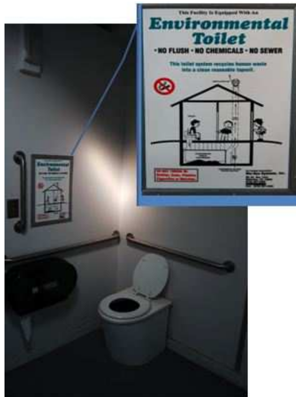
Figure 26: Interior of the women's composting toilet facility along the Schuylkill River Trail, Philadelphia
