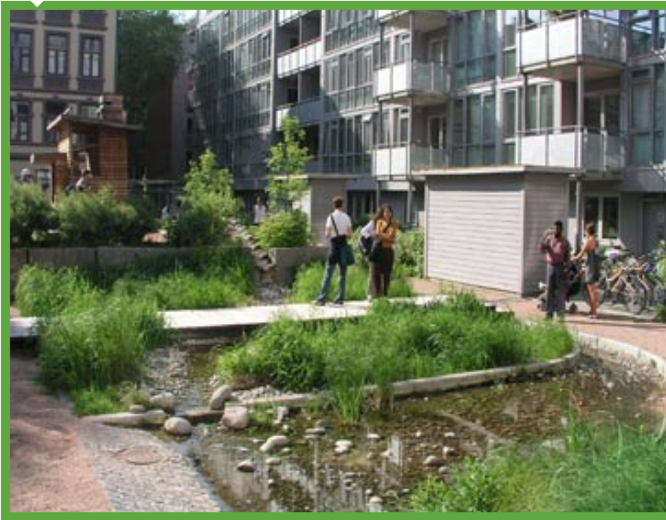
Greywater treatment using a biofilter and constructed wetland for 100 persons in Oslo, the capital of Norway. The effluent meets the current European swimming water standard with respect to indicator bacteria.
