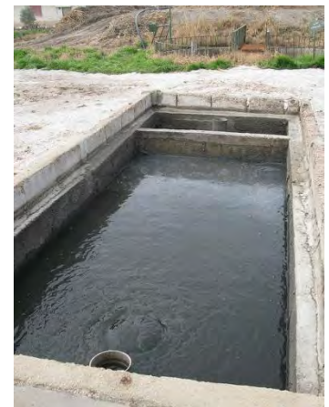
Channel for grit and fat removal
