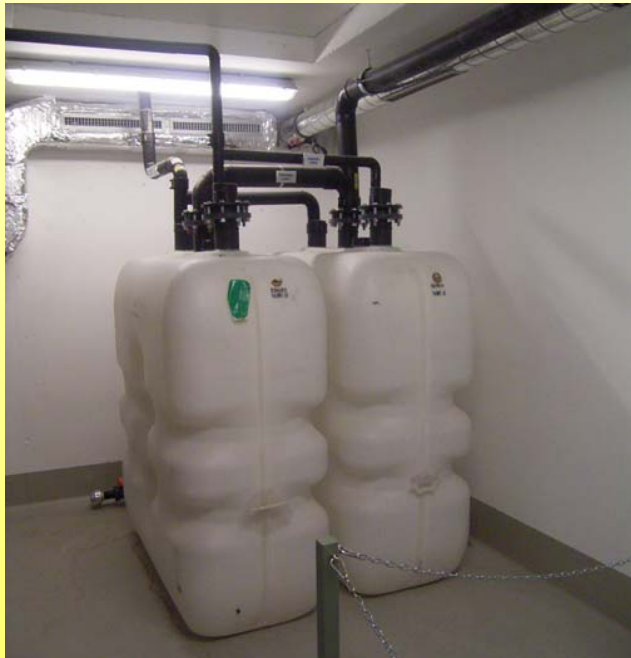
Urine tanks (photo: Otterwasser GmbH)
