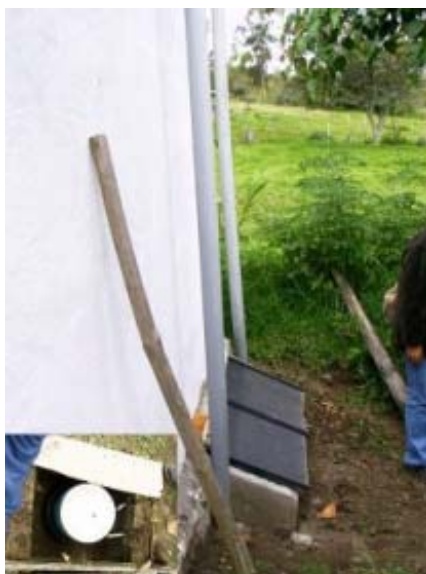
Figure 4: Storage chambers for faeces and urine storage container (photo: Xavier Zapata)
