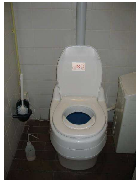
Figure 3. Installed UDD toilet in toilet cubicle for females. Note plastic squeeze bottle on the left for rinsing urine compartment.
