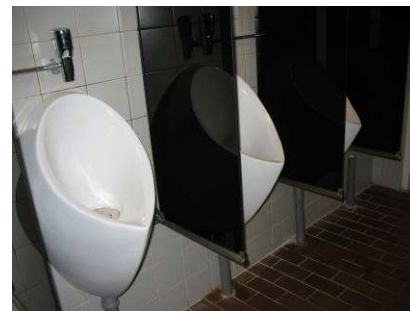
Figure 2. Installed Uridan waterless urinals
