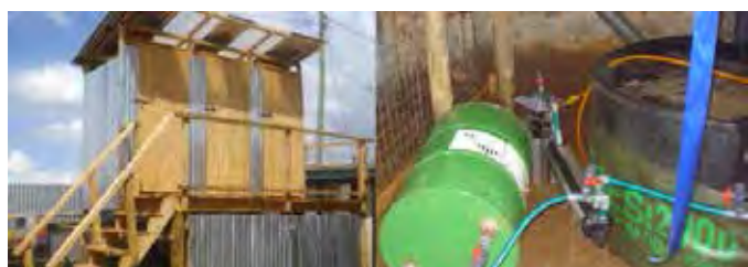
One of the three complete system and superstructure deployed in Eldoret, Kenya (left) and contained treatment system below (right). Each system comprises of three toilets, one anaerobic digester, and one heat sterilization system. All systems are self-contained.
