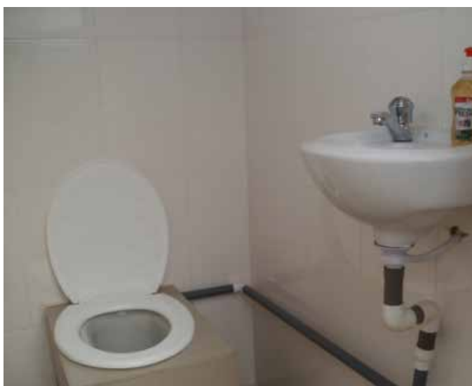
Biofil micro-flush toilet bowl plumbed to a wash basin. The grey water from hand washing creates a water seal to prevent any smell from the digester.
