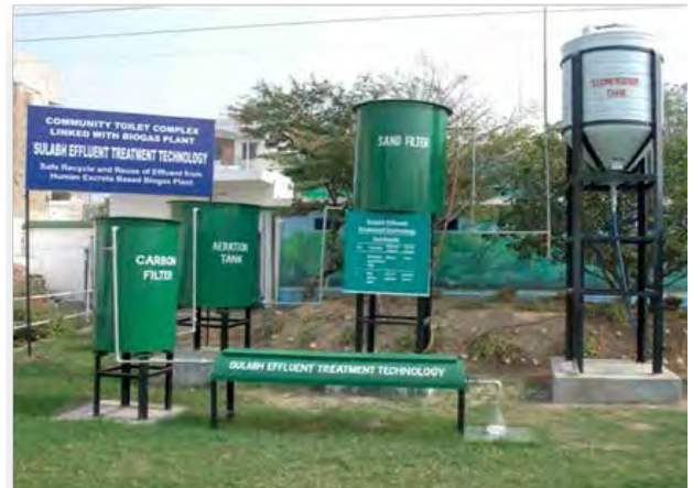
Sulabh Effluent Treatment System (SET)
