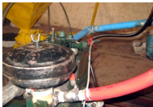
Figure 5.6 b Gas connection to the MFP
