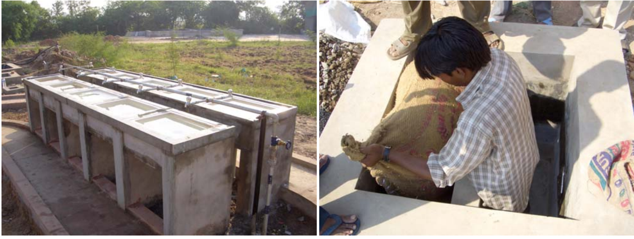
figure 9: Pic of wash-stand (left) and organic filter (right) for the treatment of water used for cleaning dishes
