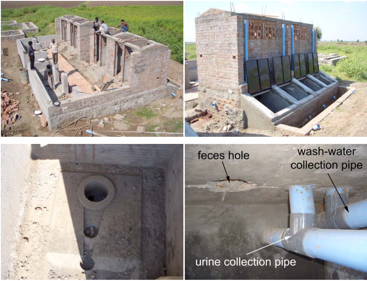
figure 11: Pic of toilet block at Navsarjan Primary School in Dhandhuka Taluka (clockwise from top left: front view of sanitation block; rear view of toilet cabins; 3-hole squatting slab; pipings for separate collection of urine and wash-water)
