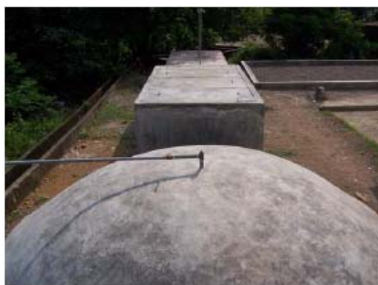
View of anaerobic treatment; digester, anaerobic baffled reactor (ABR), and anaerobic filter (AF). Gas produced from digester is piped to offal room.
