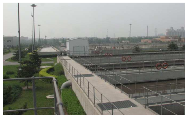
Fig. 10: Nearby Qinghe Wastewater Treatment Plant supplying irrigation water and feeding the Olympic Forest Park's waterbodies (source: Germer, 2008).
