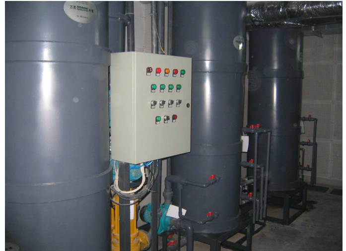
Fig. 5: Collection and storage station for the urine and brownwater (source: EnviroSystems)
