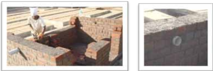
Figure 2, 3: Laying of the bricks, two pipes for ventilation to be integrated in the walls
