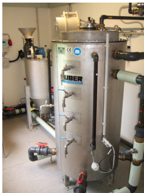
Fig. 2.4.20: Thermophile two-stage biogas plant
