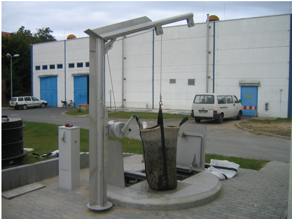
Fig. 2.4.11: Faeces dewatering facility including crane
