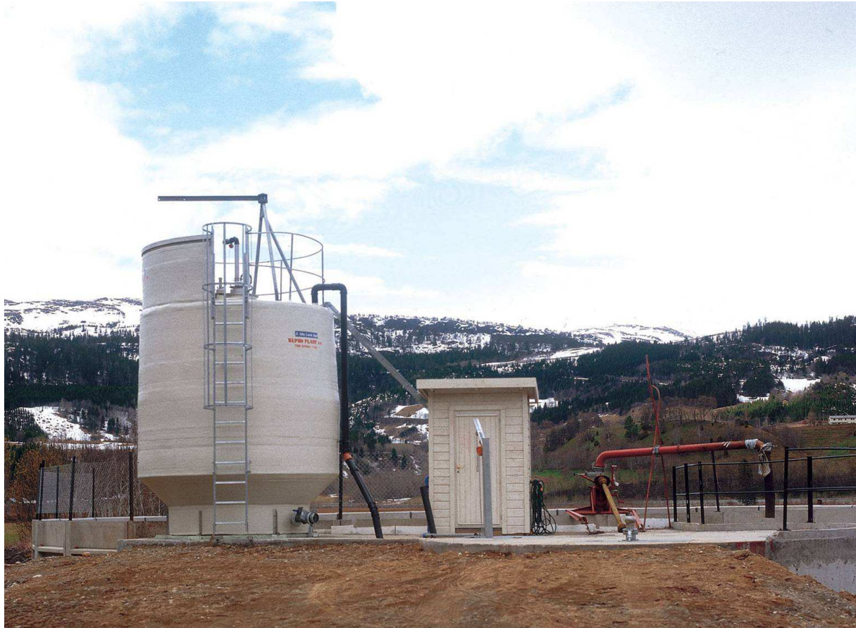
Figure 1: Liquid Composting Plant (Alva Naval) in Norway (Photo: P. Jenssen)
