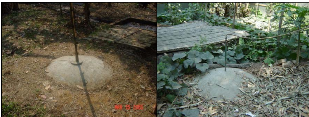
Figure 4-4 Domes were often not covered with compacted earth, outlets not covered with cast concrete slabs (right) and dome pipes always not protected
