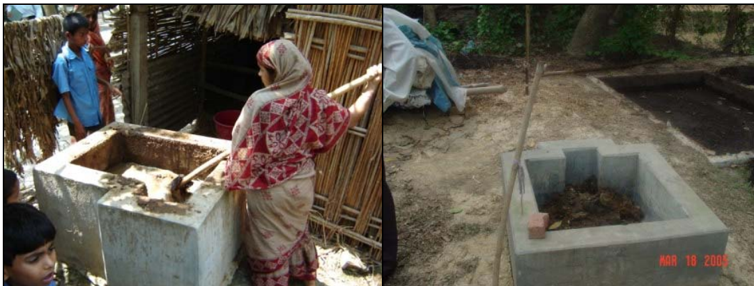
Figure 4-3 Inlets were not equipped with fixed mixing devices. The position of the inlet pipe was sometimes found 90 degrees versus the centre line (right)
