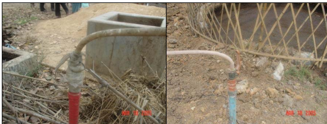
Figure 4-6 Main gas valves were sometimes wrapped in plastic (left)
