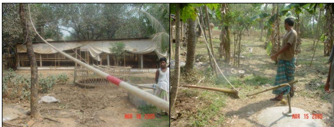
Figure 4-7 Cheap flexible plastic pipes were used to transport biogas to the place of application, sometimes poorly supported (right)
