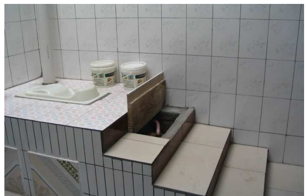
Fig. 5: Open hatch shows access to the urine pipe and urine storage tank of the UDD squatting toilet (source: Plan China)
