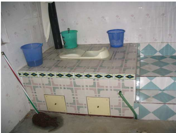
Fig. 3: Household urine diverting dehydration toilet in Shaanxi Province (source: Plan China)
