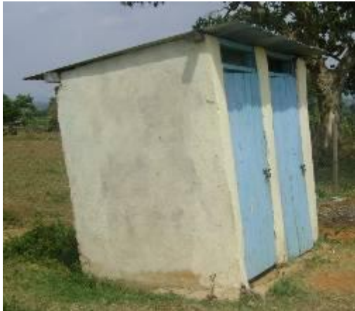
Collapsed simple pit latrine in Mumias
