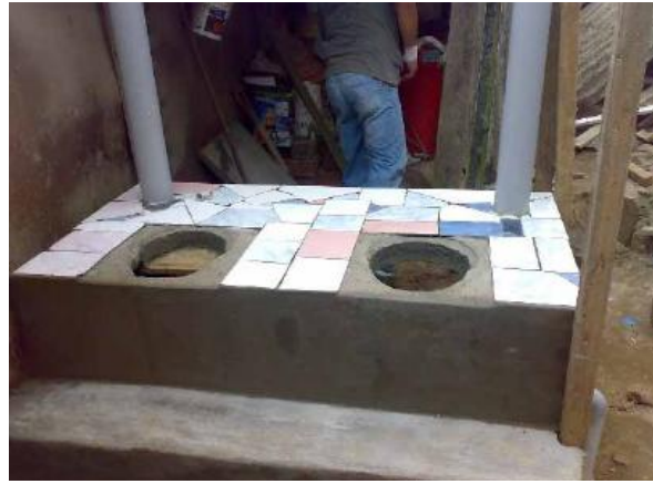
Steps, faeces chamber and toilet seats
