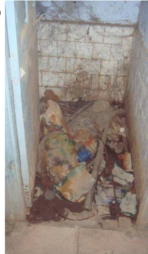
Existing toilets are in bad condition
