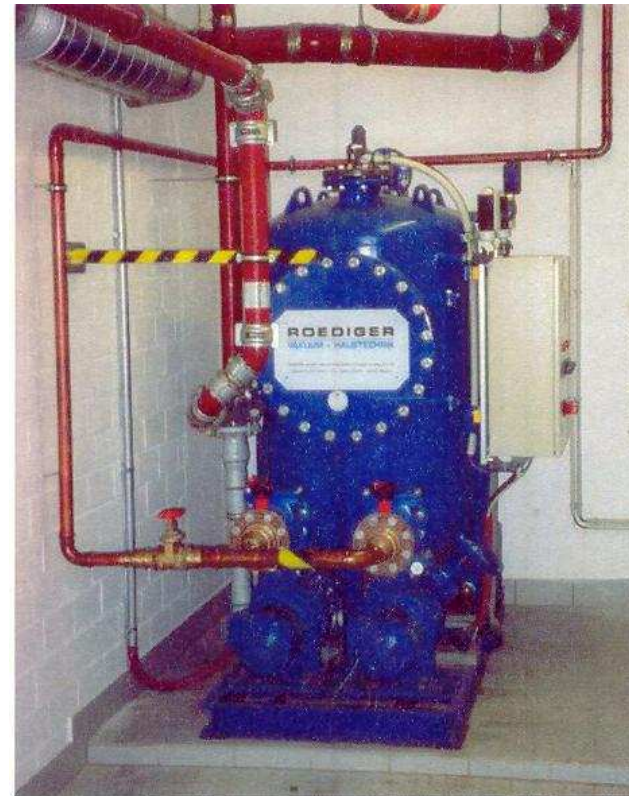
Vacuum station (pump)
