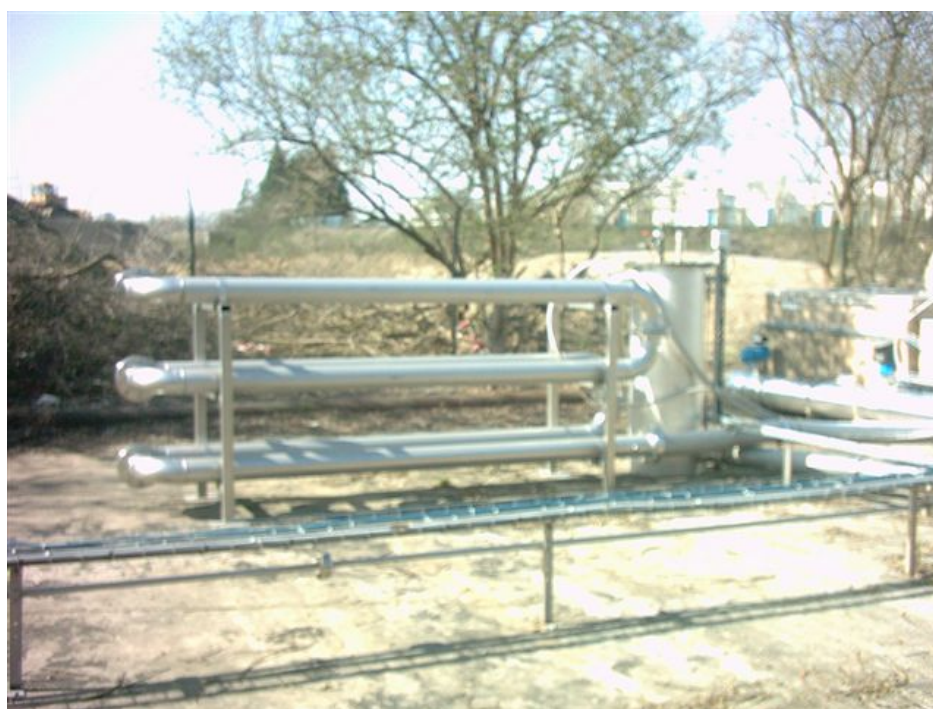
Figure 3.7: Ozonation contactor (source: Aquafin NV)
