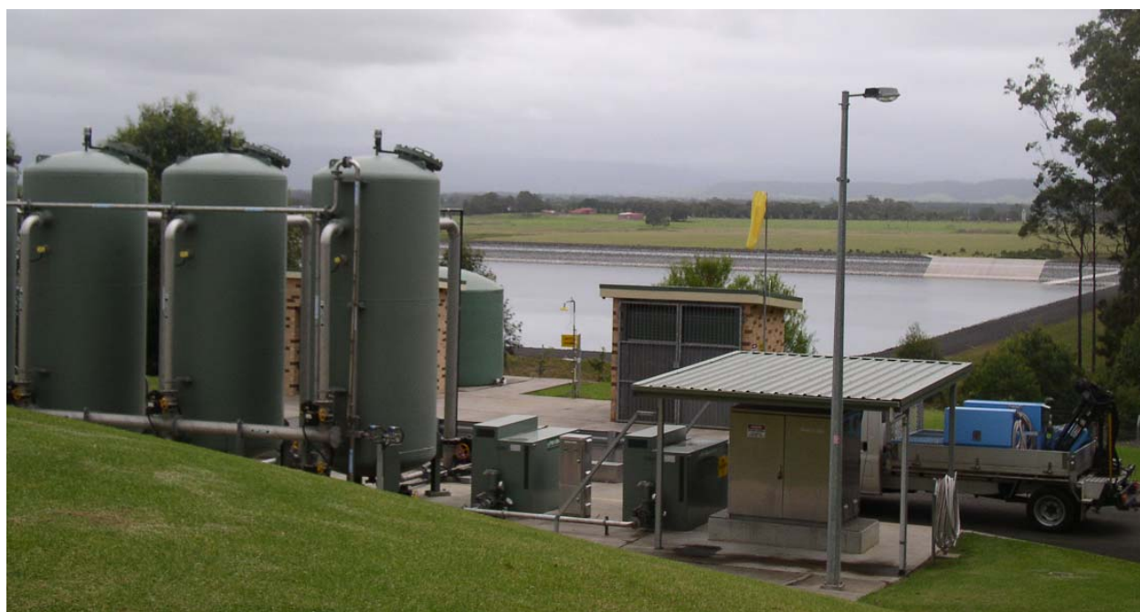
Figure 3.4: Callala WWTP Plant and Storage Reservoir [Shoalhaven Water]
