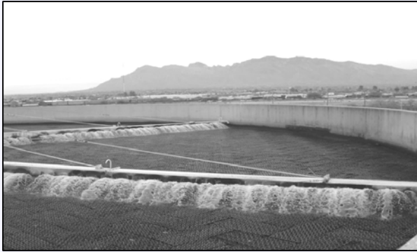
Figure 26: Tricking Bio towers at Roger Road WWTP (picture by Harm Jansen)
