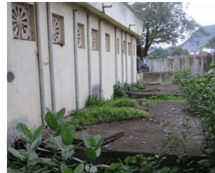
In old community toilets, septic tanks are behind the block making them difficult to access
