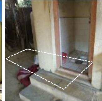
Inaccessible septic tanks with sealed tops and no access covers
