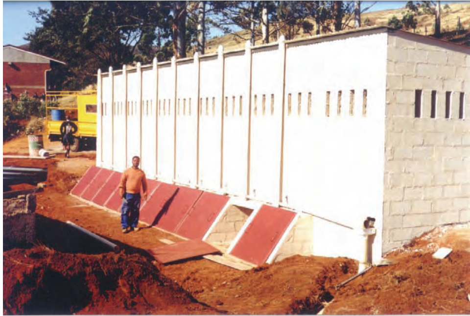
Figure 2.9: Well-fitting vault lids at a school toilet block (Photograph: CSIR)
