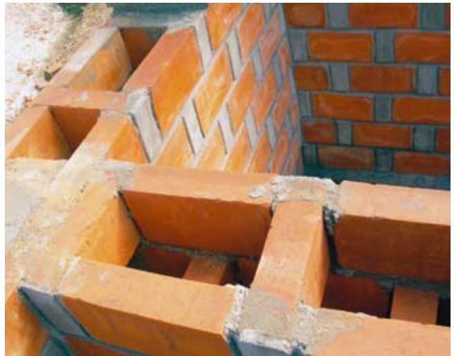
Better building methods can improve the energy efficiency of buildings: this rat trap bond masonry saves bricks and insulates better
