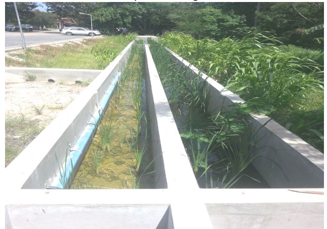
Oxidation channel in operation
