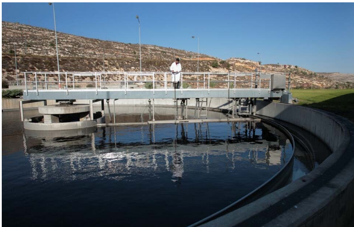
Al Bireh wastewater treatment plant (photo KfW)
