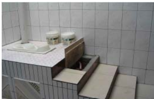
Figure 5: Open hatch shows access to the urine pipe and urine storage tank of the UDD squatting toilet (source: Plan China)
