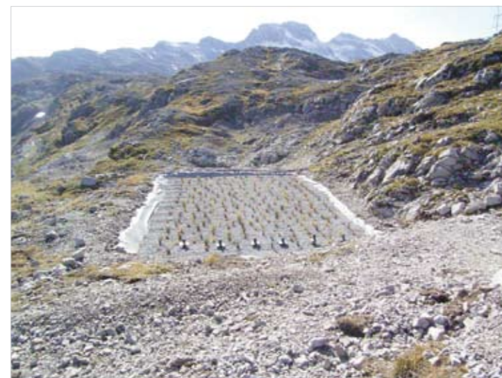
Constructed wetland for greywater treatment in mountainous area, Vorarlberg, Austria
