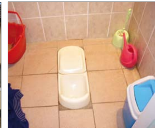
Squatting slabs inside the rest room
