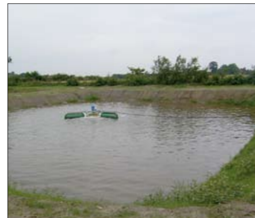
Aerated pond 3, surface aerator
