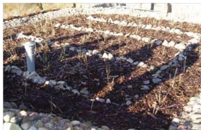
On-site constructed wetland for domestic wastewater treatment, Poland
