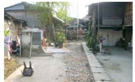
Photos 1 and 2: Different project phases, from top to bottom: An intervention plan was developed in close collaboration with the community and different interest groups (here: Village Environmental Unit defining management regulations). Construction of the stormwater drainage network.
