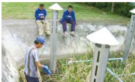
Photo 1: Constructed wetlands for FS treatment in Baan Klang municipality, Thailand.
