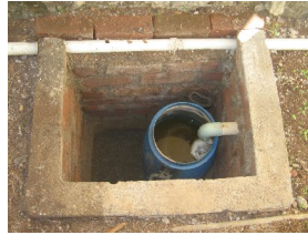
Leach pit cum holding tank with can
