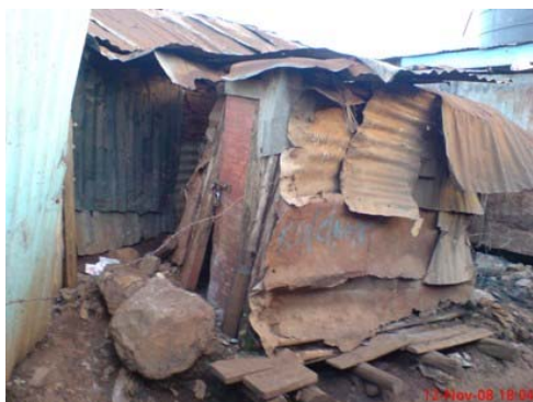
Figure 23: A poorly constructed toilet (Photo taken by author)
