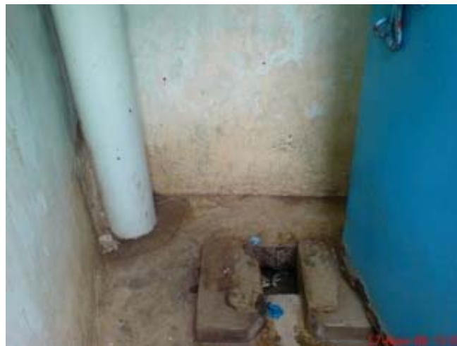
Figure 39: A biogas toilet with faeces close to platform
