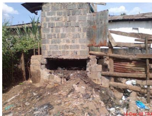
Figure 24: A hanging toilet (Photo taken by author)
