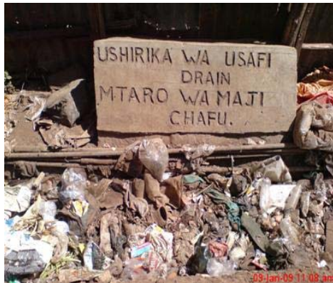
Figure 5: Drainage channel full of solid waste (Photo taken by author)
