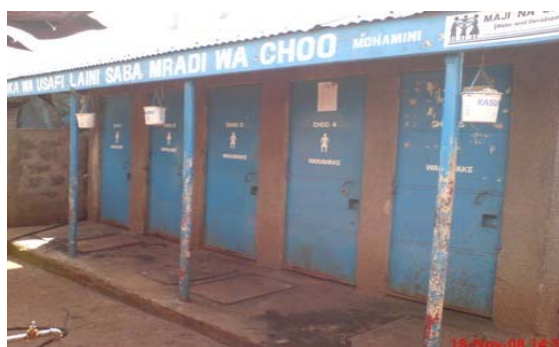
Figure 12: The selected Soweto VIP toilet (Photo by the author)
