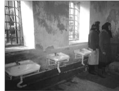
The wash basins installed in a school in Garla Mare.
