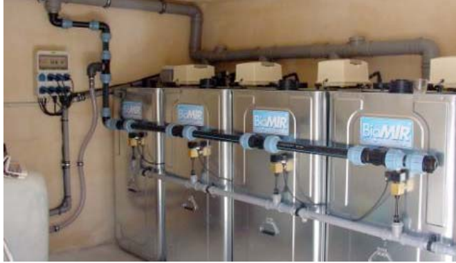
Biomembrane reactor for high-tech decentralised wastewater treatment
