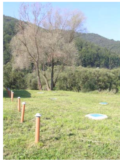
IchyPotok – (150 EO) – reconstruction of septic tank + underground sand filter, 3 water cascades with fish. System works without electricity
