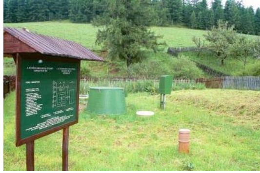
Nizné Repase (25 PE) 3 steps on site WWTP for 5 houses (septic tank, biofilter wetland for summer time and sand filter for winter time)
