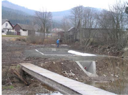
Nálepkovo – Zadny Hámor – 2007 (5 houses) Constructed wetland as a second step of treatment, first time approved in Slovakia 3-compartment septic tank and wetland, system works without electricity
