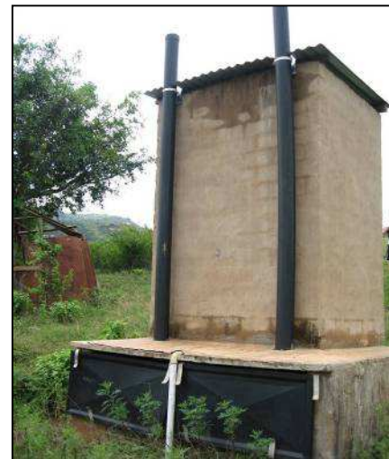
Fig. 7: Back view of double vault UDDT showing access doors to two vaults and ventilation pipes (source: EWS).
