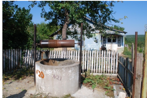
Figure 21 An unimproved dug well (missing both cover protection and apron slab).
