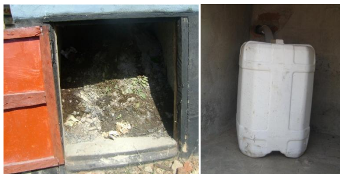
Fig. 5: Toilet chambers almost full Fig. 6: Urine canister
