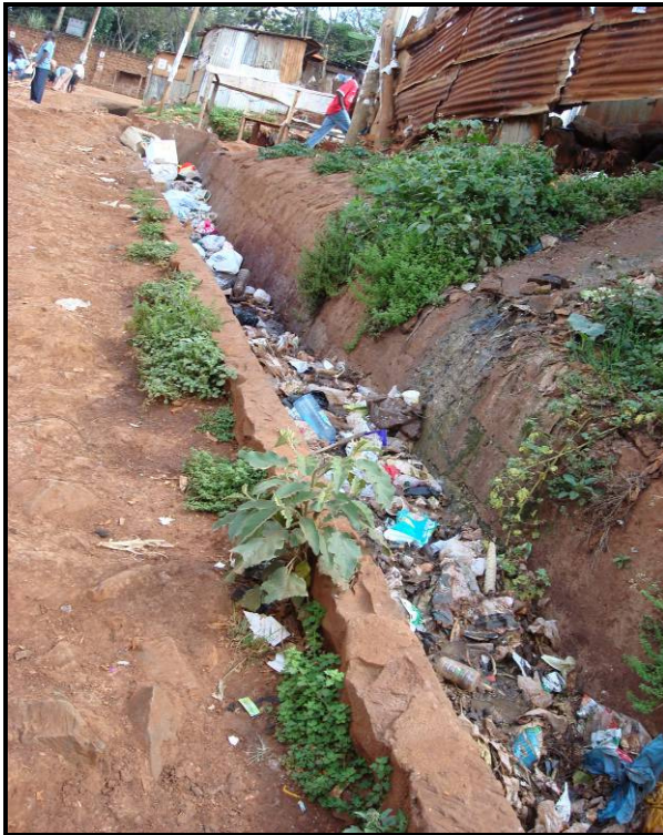
Figure 4-6: Greywater draining to solid-waste filled stormwater drain in Waruku
