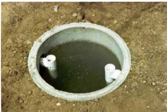
Figure B17.1: Grease interceptor
