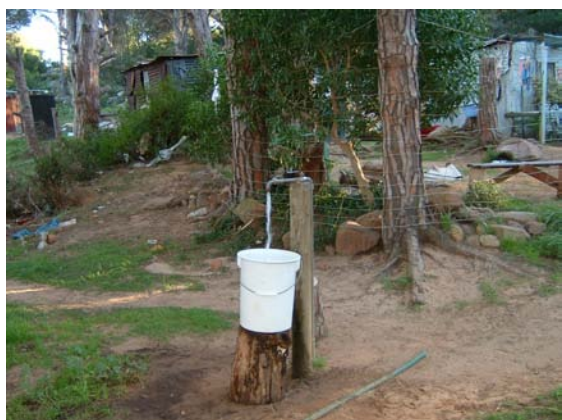
Figure D1.4: Tapstand at Redhill
