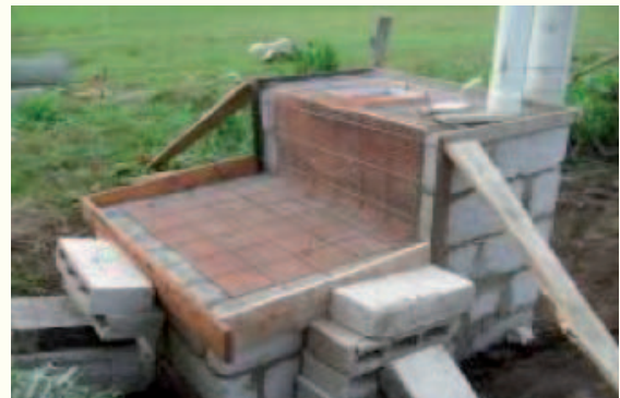
Figure 2: Ferrocement floor and bench before adding concrete. The brown plank forms have no need for holes. (Photo: C. Thibodeau)
