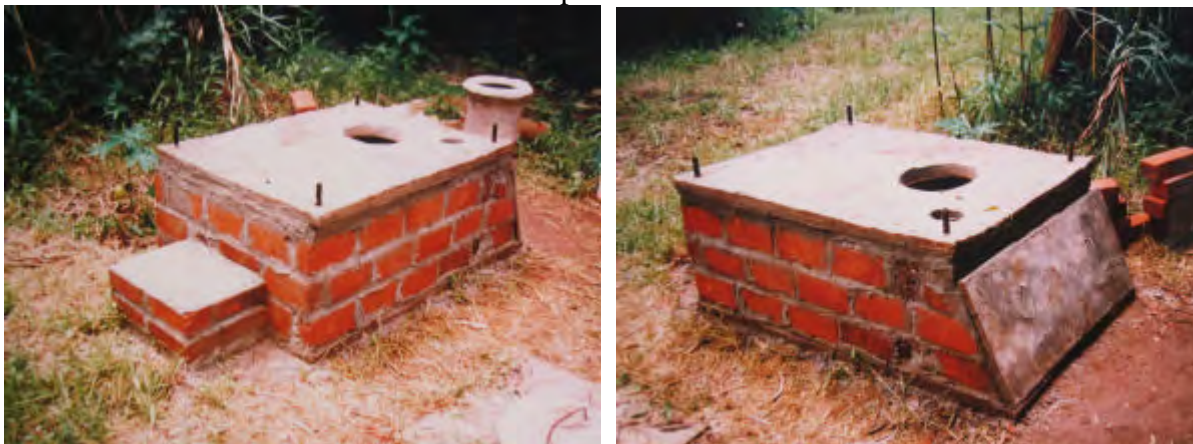
The vault access slab and the toilet slab have now been fitted. The superstructure must now be made.
