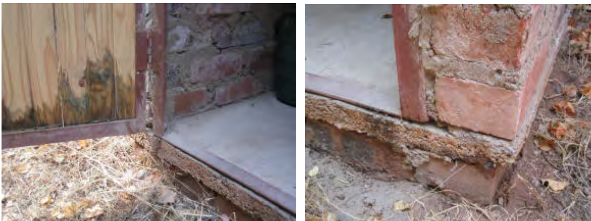
Closer views are parts of the frame. In this case the frame is made from 40mm X 40mm X 5mm angle iron. In this case the hinges are steel, but a more durable hinge can be made from car tyre. This is shown in the chapter on special construction techniques later in this book.
