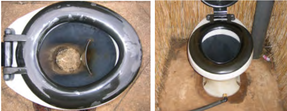
This urine diverting pedestal has been fitted to a Fossa alterna system. The urine off-take is fitted above the base of the pedestal so that the pipe can be led above the slab to the most suitable place – like a container, compost-pit or tree. The 110mm vent pipe passes through a hole made in the slab and is fitted in this case inside the toilet house.
