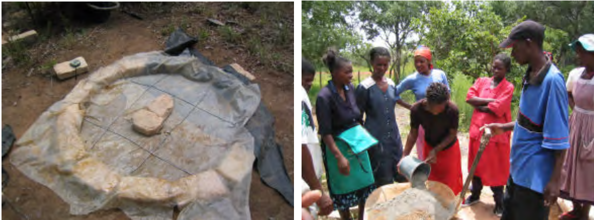
Plastic sheet is placed inside the mould and the concrete mix is made up in a wheel barrow (30 litres of good clean river sand and 5 litres of fresh cement. This is thoroughly mixed before and after adding water to make the concrete mix. Using this economy mix 8 slabs can be made with a single 50kg bag of cement.
