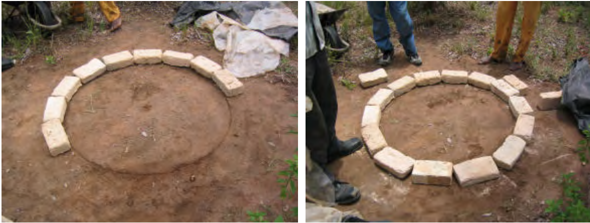
The circle for the 1 metre diameter slab mould is marked on levelled ground and bricks placed together in a circle
