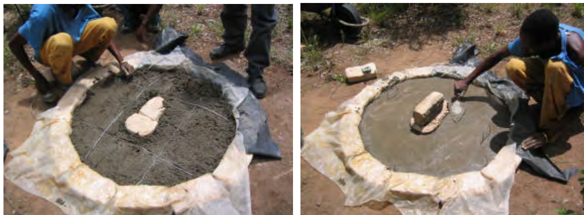
A mould for the squat hole is made with a bucket or with bricks as shown here. Half the mix (about 17 litres) is added to the mould first and levelled off. The four 90cm pieces of wire (3 – 4mm thick) are added to make a wire square around the squat hole. Then the remaining concrete is added, levelled, tamped down hard and finished off with a wooden float and steel trowel.
