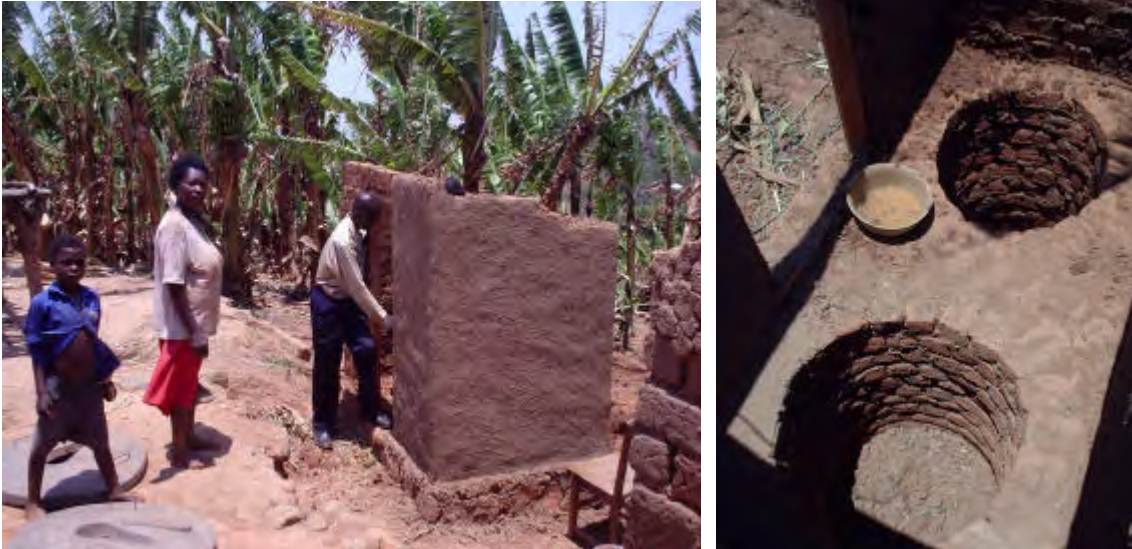
On the left a permanent brick Fossa alterna structure is built around two brick lined pits in Thyolo, Malawi (COMWASH Project). The brick lined pits are shown on the right.
