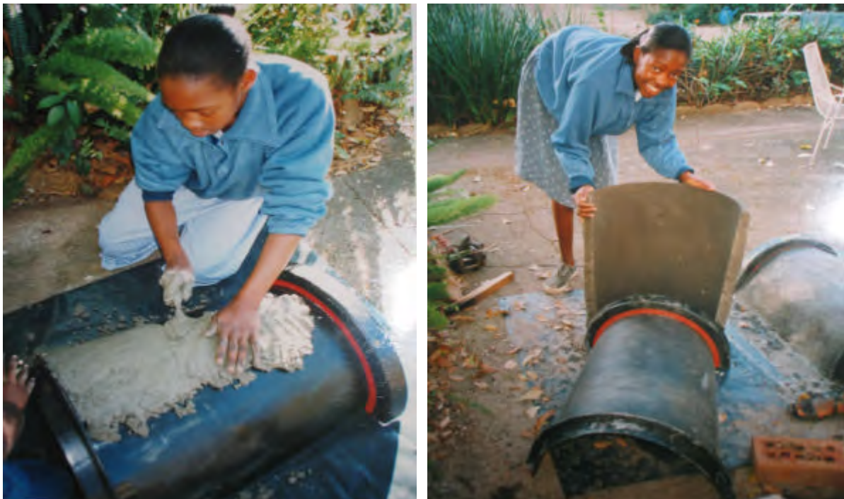
Making the larger 80 litre split cement jar using a plastic dustbin as a mould.
