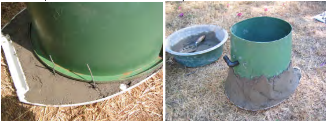
8 pieces of bent wire are now introduced into the cement supporting the seat. This is allowed to cure overnight. Next a further mix of 3:1 sand and cement is made and plastered half way up the walls of the bucket. This is left overnight again to cure.
