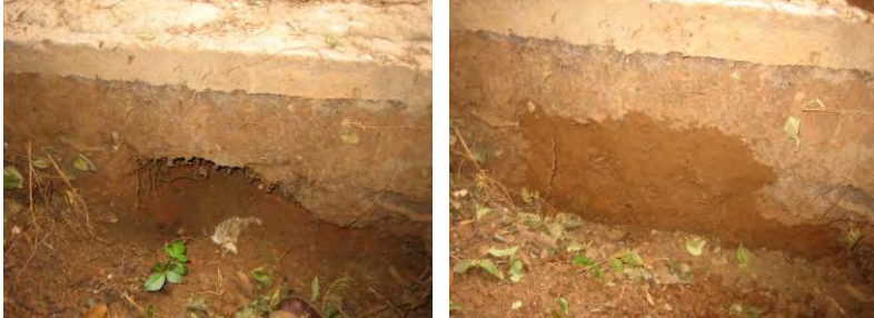
Photos showing eroded section of pit wall under ring beam. This has been filled with a mix of red soil and cement to stabilise.
