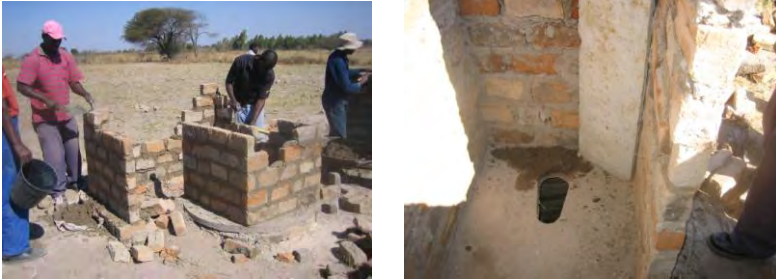
Brick walls are built up. In this photo the pipe was made with a concrete panel mounted on interior wall over vent hole.
