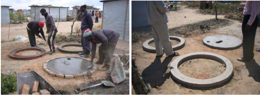
Two ring beams and a single slab are cast for the alternating pit system
