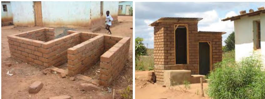
Double vault system being built in Lilongwe, Malawi. In this case the toilet is coupled with a washroom. Programme by CCODE Malawi.
