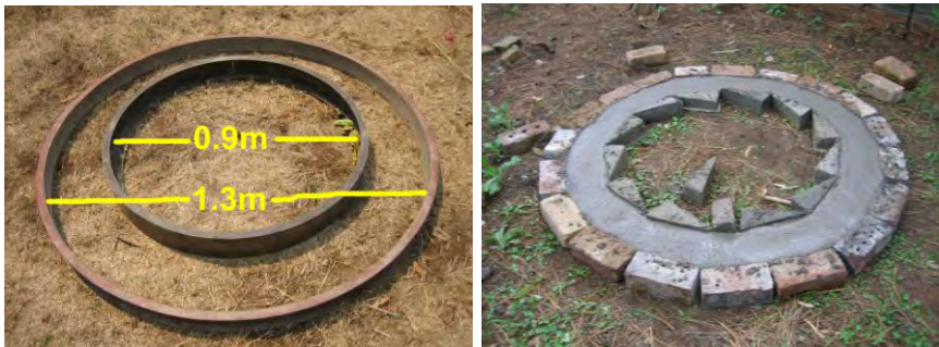
Figures 3 & 4: Both steel and brick shuttering can be used to make the ring beam.
