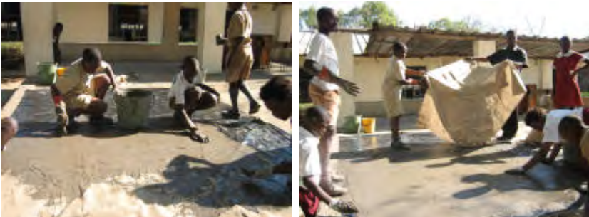
Adding cement paint to the first layer of hessian. Adding the second layer of hessian, once the first layer has been filled with cement.
