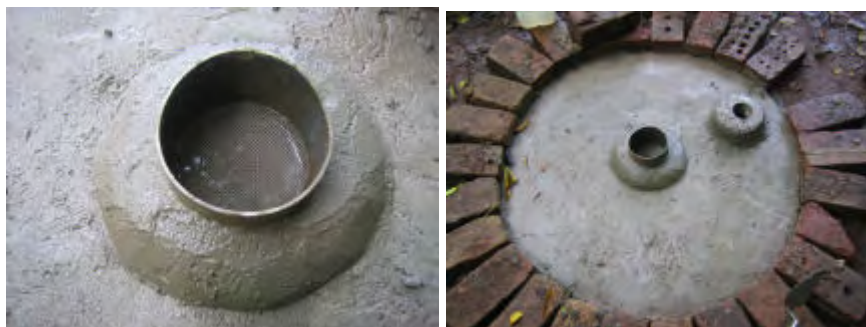
Central hole of upper tank slab with stainless steel screen and also the concrete plate made to hold the 50mm steel pipe socket in which the hand pump (Blair Pump) is screwed.
