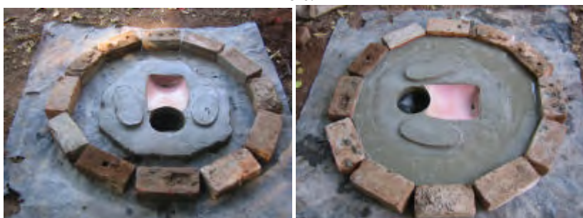
A circle of bricks is laid down around the slab to the required size. This is then filled with concrete with some reinforcing wire inserted. It is left to cure.
