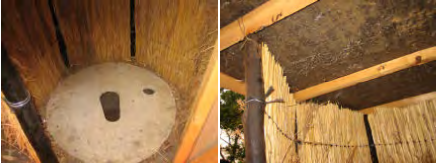
The slab inside the toilet house. At first a pipe may not be fitted. The pipe can be fitted later. When plenty of soil and ash are added to the pit smells and flies are reduced.
