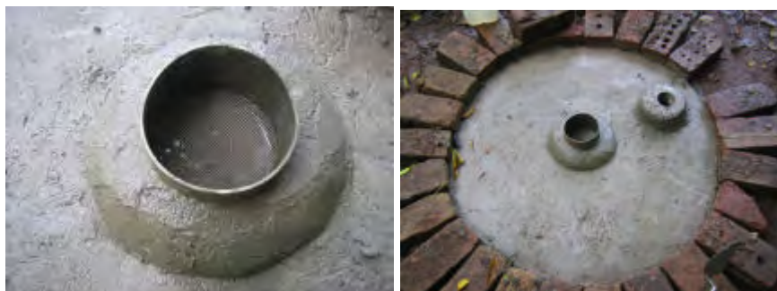
Central hole of upper tank slab with stainless steel screen and also the concrete plate made to hold the 50mm steel pipe socket in which the hand pump (Blair Pump) is screwed.
