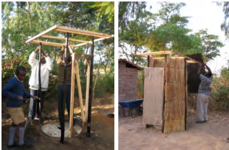
Attaching the frame to the simple treated gum poles structure. And adding the cement filled hessian sheet to the frame.
