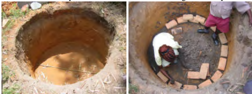
In this case the pit was dug 1.5m across and 1m deep. A mix of one part cement and 15 parts pit sand was used to make the cement mortar.
