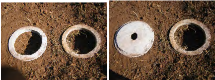
Two ring beams used in the Fossa alterna . Cast ring beams in place and when hard dig inside both down to 1.2 to 1.5m. Add a sack of leaves to the pit which be used. Fit the slab on one ring beam and cover the second for safety. The second can be filled with leaves and soil to make compost.
