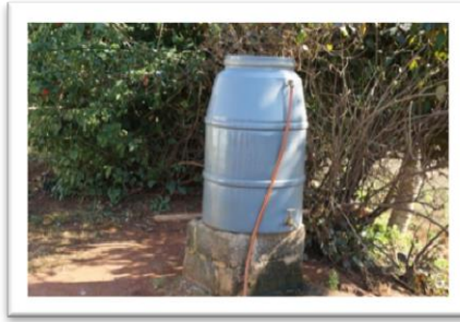
Figure #17: A 200L above ground water tank supplied by municipality
