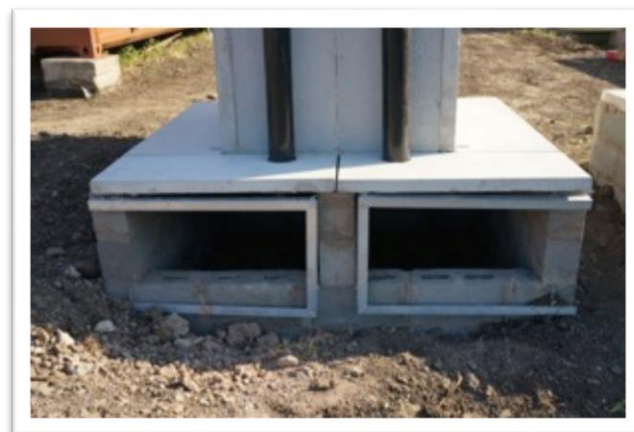
Figure #4: Inside of a VIP toilet. The toilet has a urine diversion partition in the front (red arrow) which drains into a bucket partially buried to the rear of the VIP. As presented the second chamber opening connection is shown to the left of the toilet. After six months the toilet is moved to the new port by the resident.
