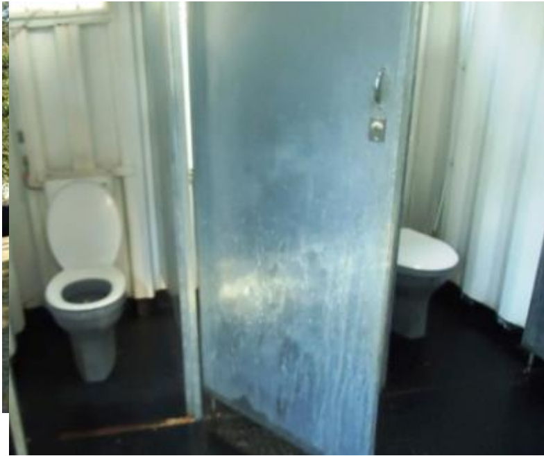
Photograph 1: One of 3 ablution blocks in the Fraser Settlement. eThinkwini Municipality in the Province of KwaZulu-Natal.
