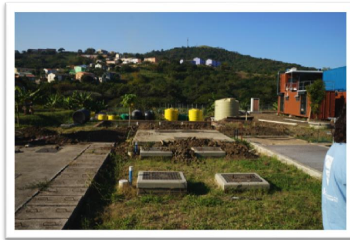
Figure #3: The DEWATS Demonstration Plant
