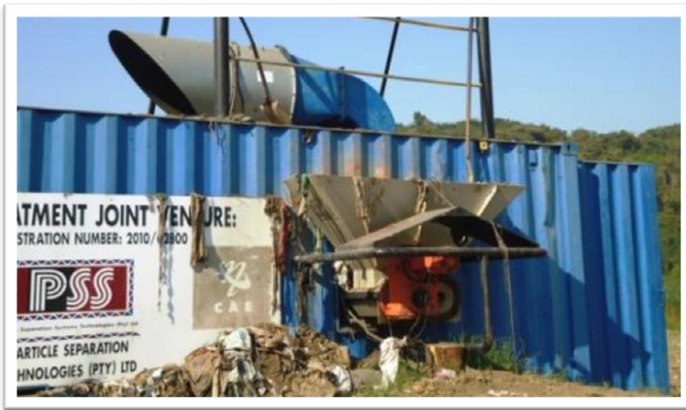
Figure #11: The grinder removes garbage from the solid waste before it is processed in the LaDePa.
