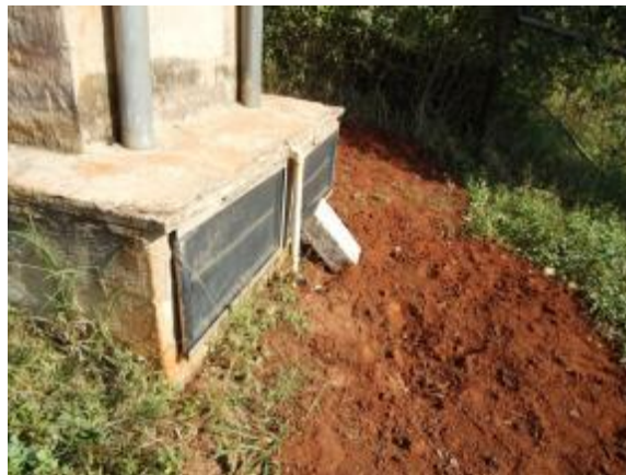
Photograph 6: The back of the urine diversion toilet. Each panel on the back represents where the waste for each hole goes to.
