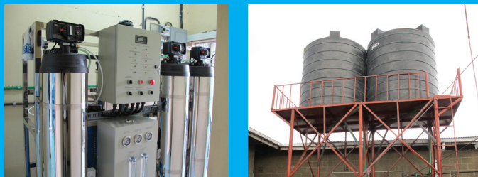
Advanced treatment system at a vended water business. Right: Storage capacity allows vended water businesses to avoid supply disruptions.
